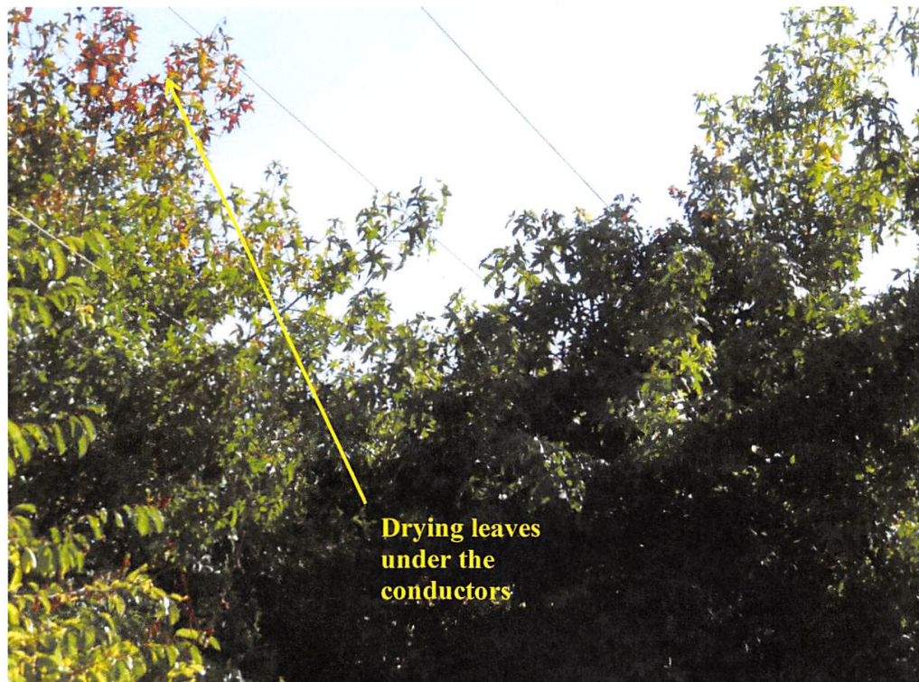
Figure 12. Example of a 12 kV line with tree limbs approaching the conductors
