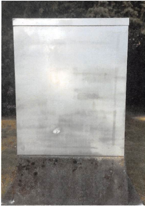
Utility Box at Rhododendron Park
