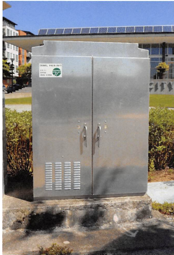
Utility Box at City Hall
