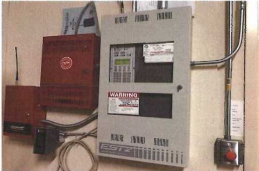
#31 FIRE ALARM CONTROL PANEL
