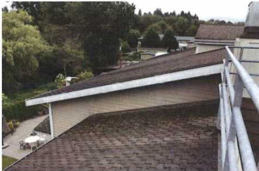
#7 ROOF VEGETATION GROWTH - REQUIRES CLEANING
