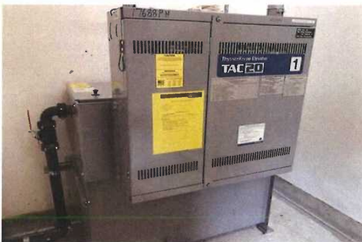
#17 HYDRAULIC ELEVATOR MACHINE
