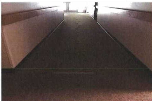
#11 DAMAGED CARPETING IN HALLWAY
