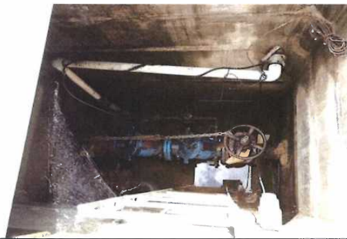
#26 FIRE SUPPRESSION BACKFLOW PREVENTER
