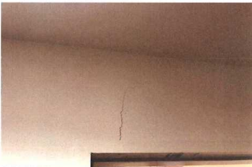
#5 SETTLEMENT CRACKING ABOVE DOORWAY
