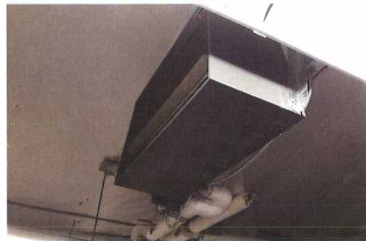
#22 UNIT HEATER IN MECHANICAL ATTIC
