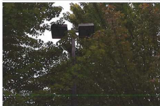
#30 EXTERIOR LED LIGHTING
