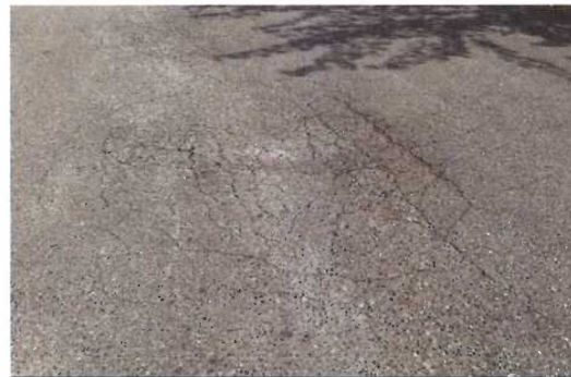
#46 ALLIGATOR CRACKING IN PARKING LOT
