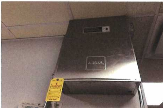
#27 KITCHEN SUPPRESSION SYSTEM
