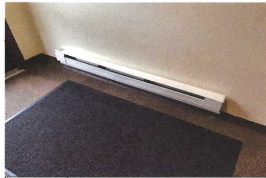
#38 HALLWAY ELECTRIC BASEBOARD HEATER
