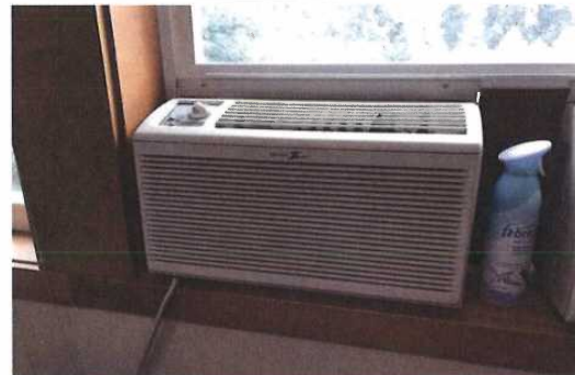
#24 WINDOW AIR CONDITIONER
