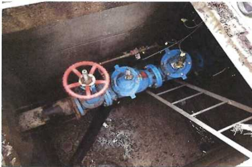
#39 FIRE PROTECTION BACKFLOW PREVENTER
