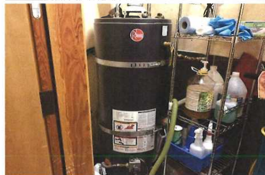
#30 DOMESTIC WATER HEATER
