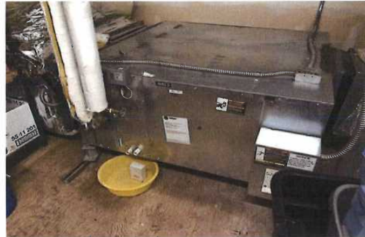
#20 INTERIOR AIR HANDLER
