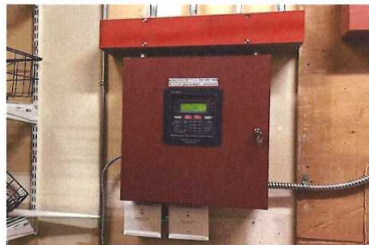
#42 FIRE ALARM CONTROL PANEL
