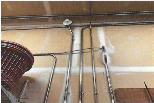
#43 NEW FIRE ALARM COMPONENTS
