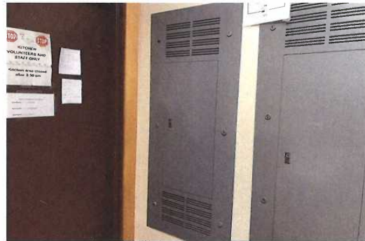
#40 ELECTRICAL PANELS IN KITCHEN
