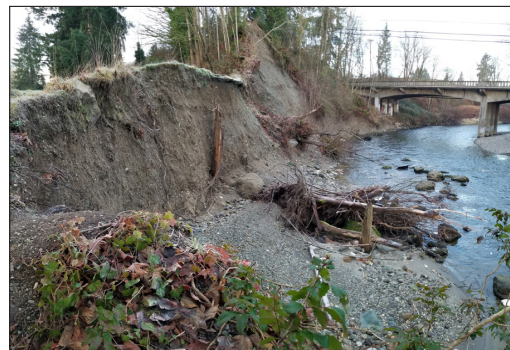
Pilchuck Park River Erosion; Snohomish, Washington
