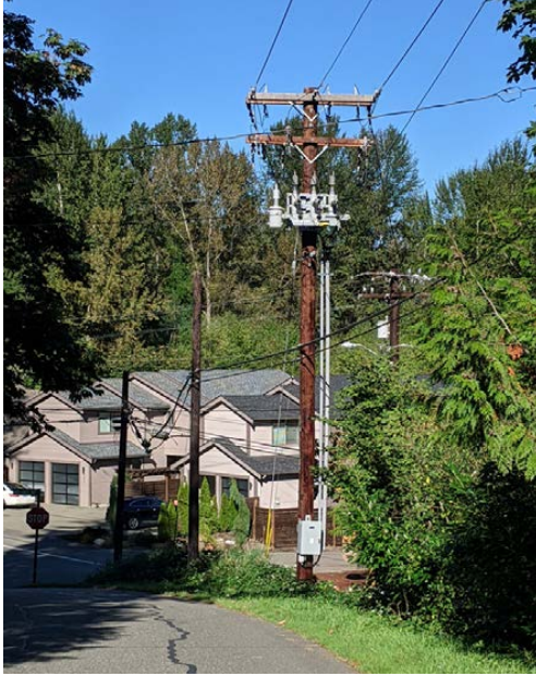
New Smart Recloser
