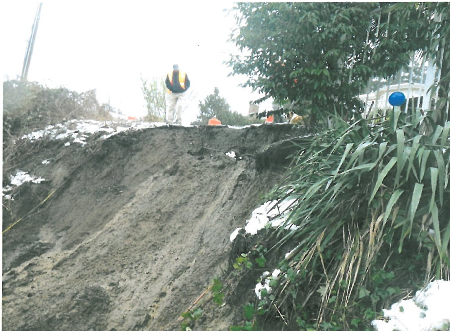
Photo #6: Top of slide area from 15219 NE 61 st Place NE (facing north-east)
