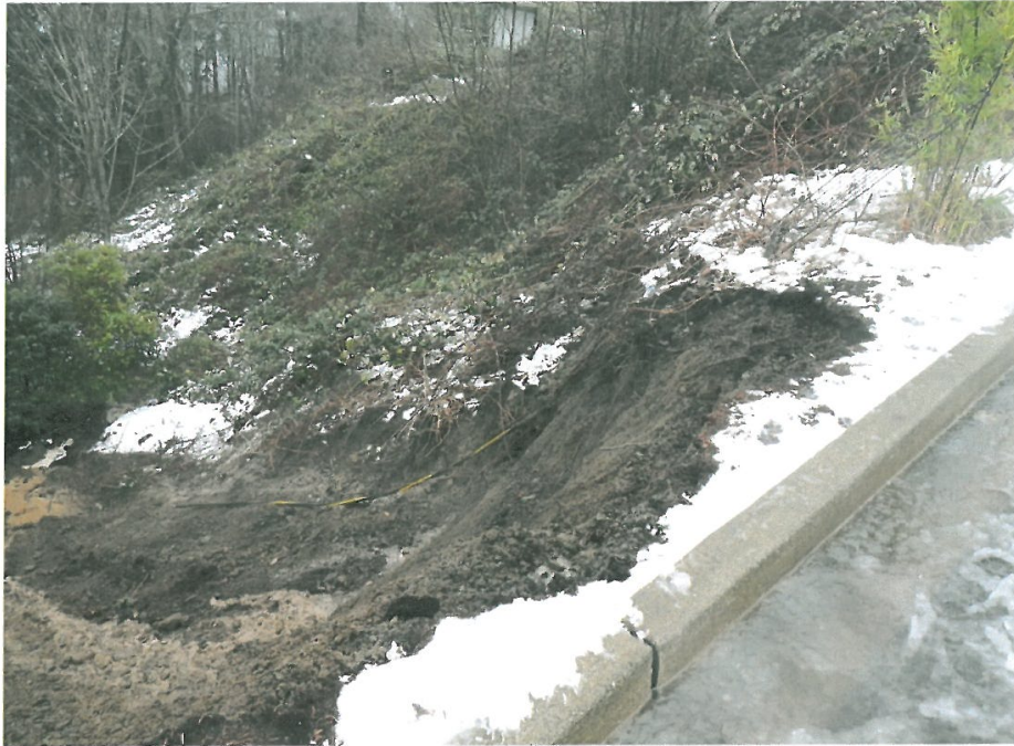
Photo #7: Top of slide area from 61 st Place NE (facing north-west)
