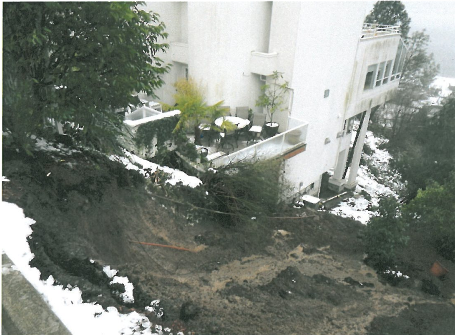
Photo #8: Slide area from NE 61 st Place NE (facing south-west)
