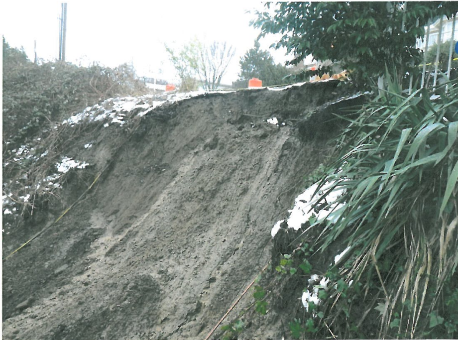
Photo #4: Slide area from 15219 NE 61 st Place NE (facing north-east)
