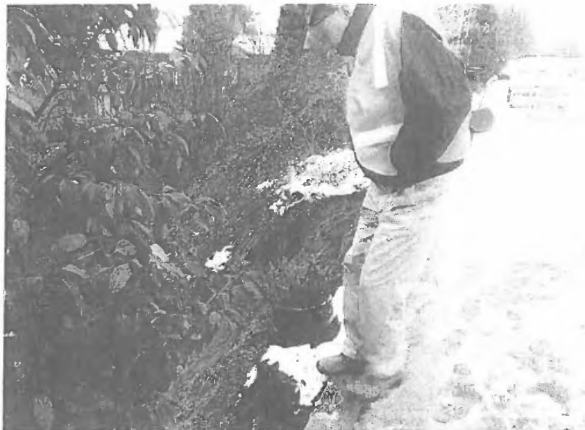
Photo #2: Top of slide area from 61 st Place NE (facing north)
