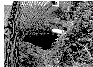
Undercut sidewalk at NE 190 th St.
