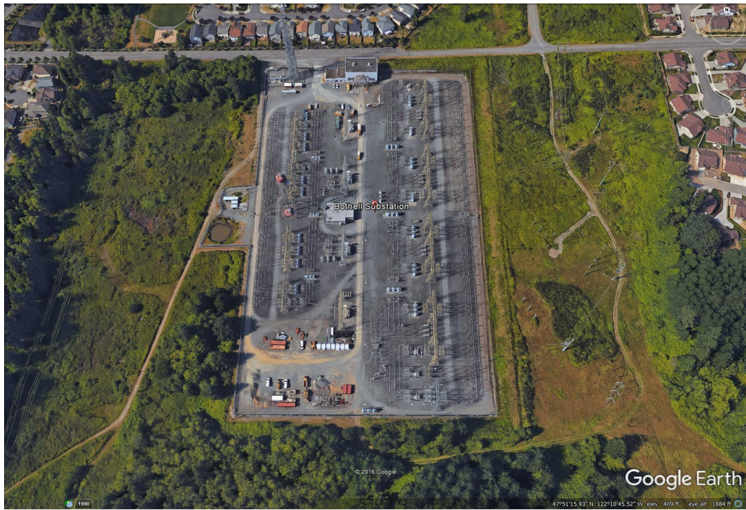
Figure 7. The Bothell substation.
