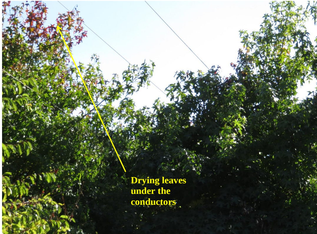
Figure 11. Example of a 12 kV line with tree limbs approaching the conductors
