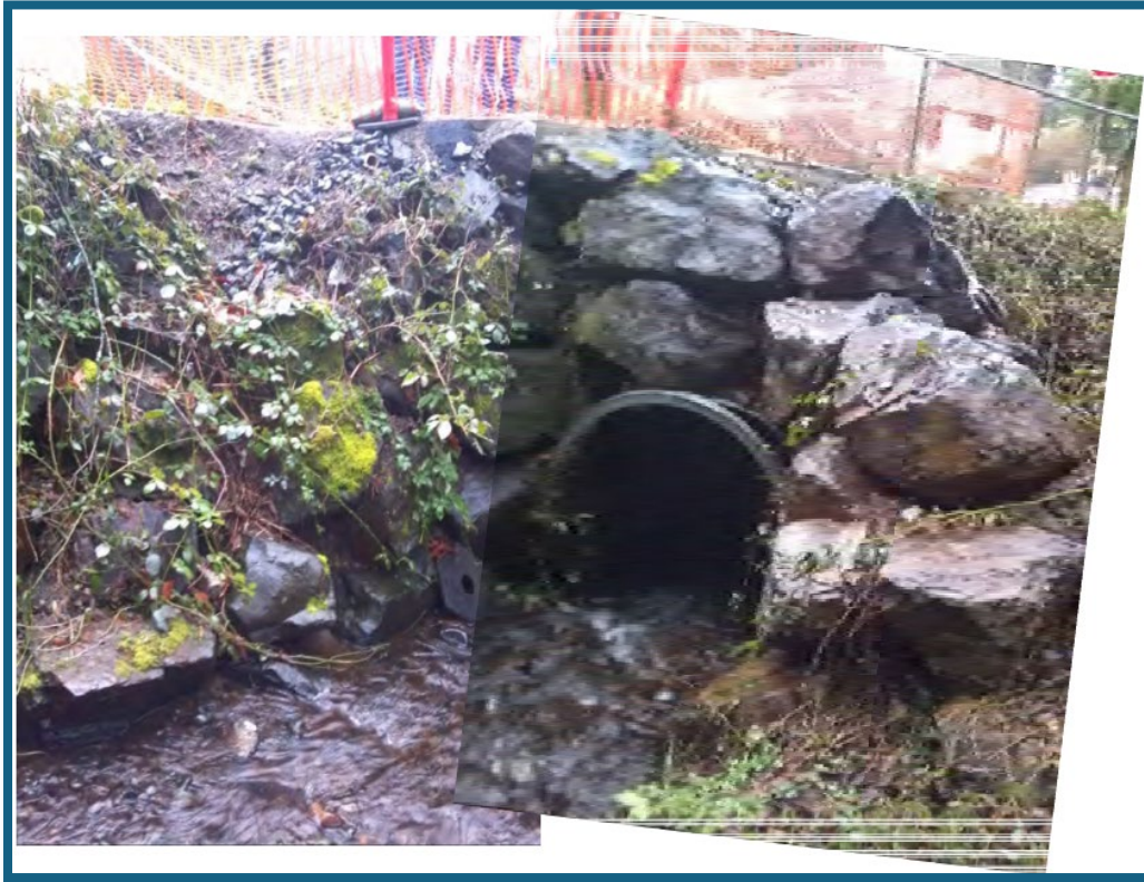
NE 190 th St Preexisting (failing) Culvert
