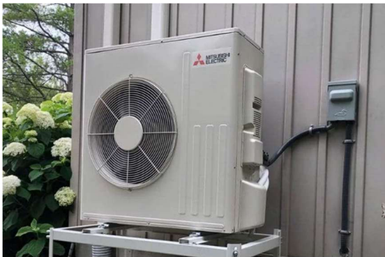
Example of typical heat pump install
