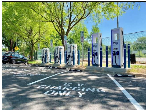
Example pull-in EV charging stations.
