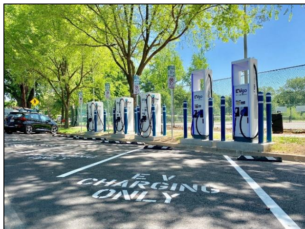
Example pull-in EV charging stations.
