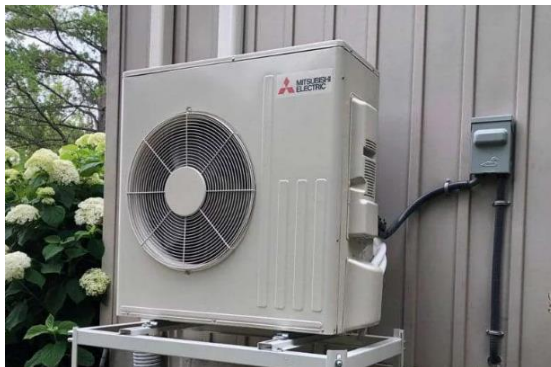
Example of typical heat pump install
