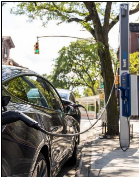
Example curbside EV charging stations.
